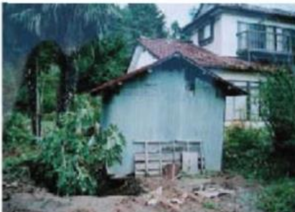
(b) 陥没穴と噴砂
