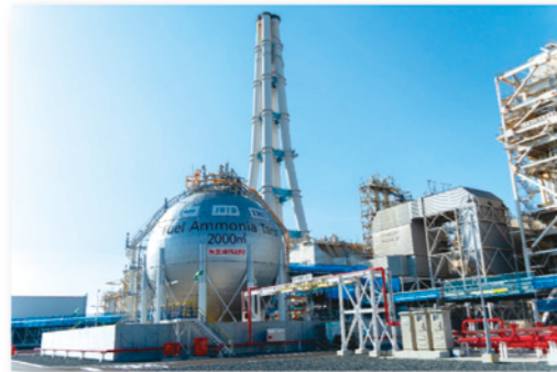
JERA Hekinan Thermal Power Plant aiming for substitution to ammonia fuel
